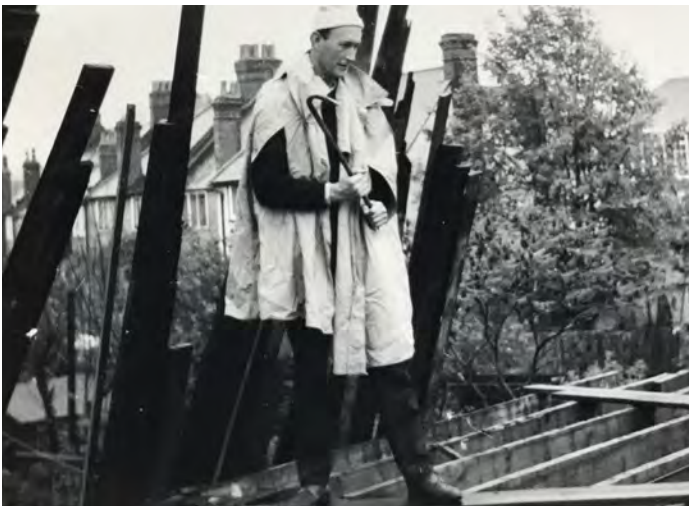
Demolition on site - Myles apparently wearing improvised hi-vis on the roof of the old clubroom.
